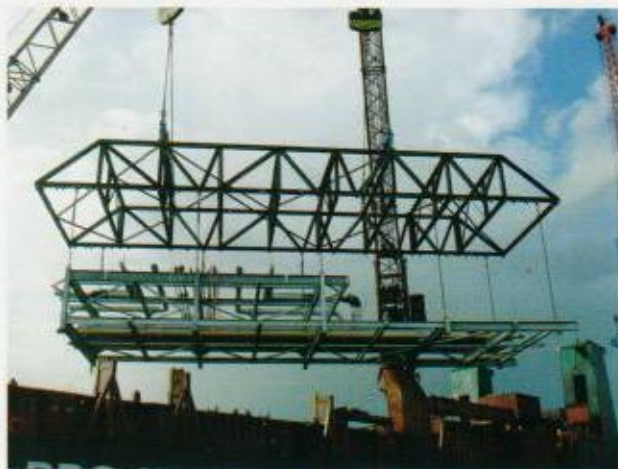
Figure 3. A crane is used to hoist the pre-fabricated pipe to transport it for module construction.
